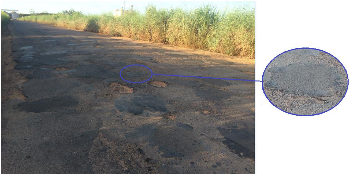
Figura 38: Remendos - Rodovia TO-070.
